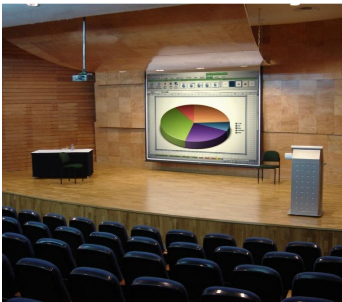
TecPodium All in One Multimedia Lectern installed at the 300 seats prestigious Auditorium
